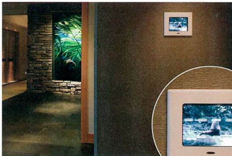
Vantage touchscreen controls are placed throughout the house in areas needing the most control. Simple and intuitive total home control is possible thanks to programming designed for first-time users.
