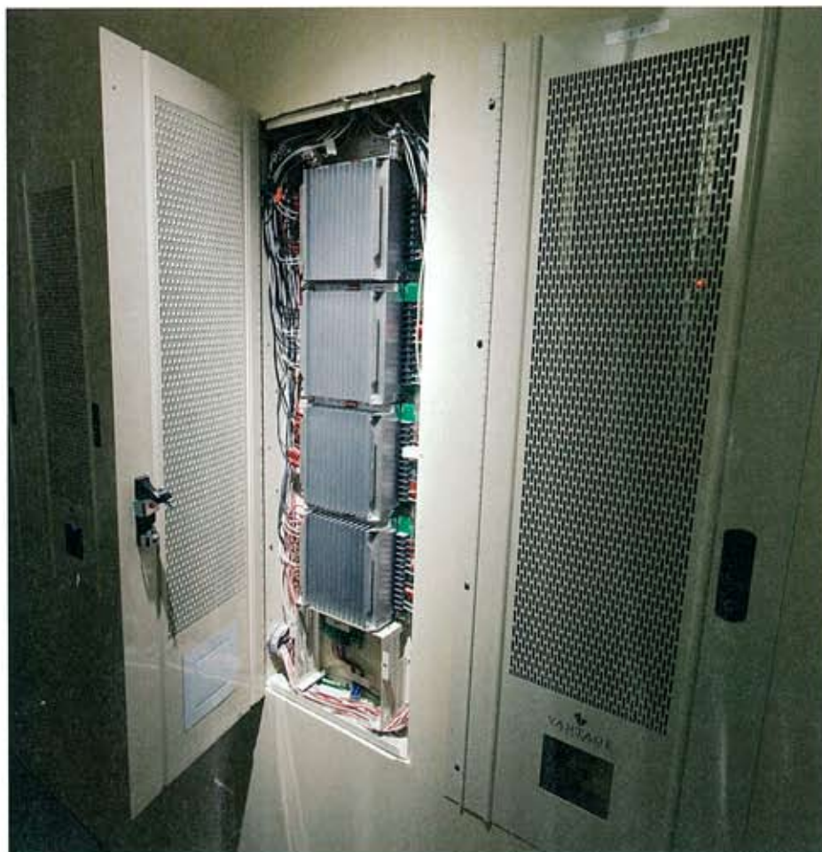
An entire wall in the electrical equipment room is needed to house all the panels required for the multitude of home technology systems integrated in this home. The electrical contractor stumbled upon this dead space and claimed it for the electrical equipment.
